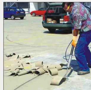
Peeling of 2-component coatings
