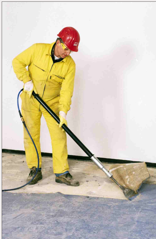
Loosening of linoleum
