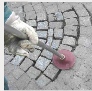
Blow out joints
